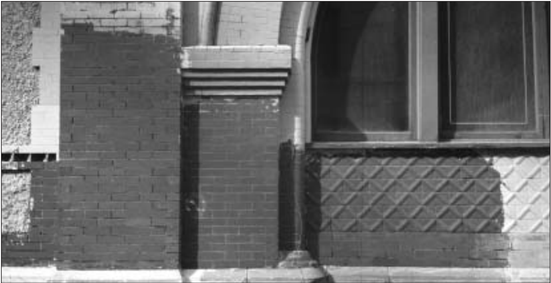
Renovation extends a building's service life, reducing the use of new materials.
