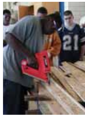
Figure 13a Students at the Max Hayes Vocational High School in Cleveland, Ohio build prototype SEE studs as part of the process of gaining builder and building official approval for SEE stud use in the Building America project, EcoVillage Cleveland townhomes at 58 th St.
